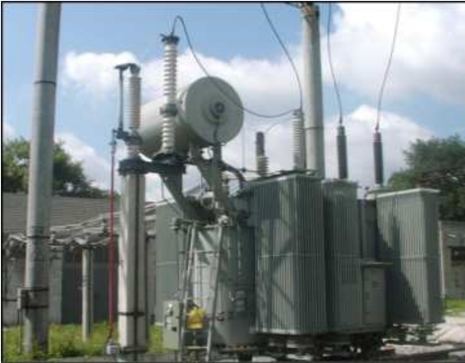
Figure 2. The The Power transformer at the Substation after the reconstruction
