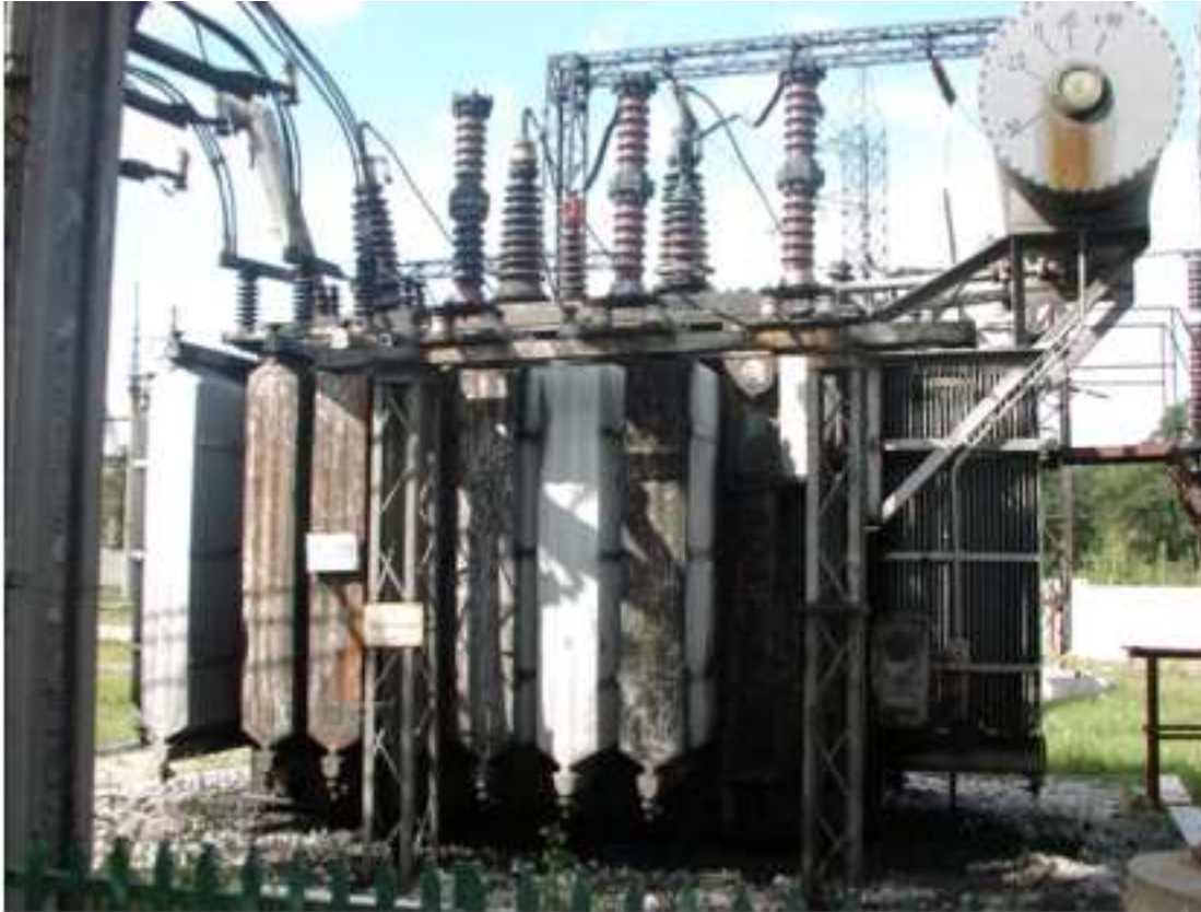
Figure 1. The Power transformer at the Substation before the reconstruction
