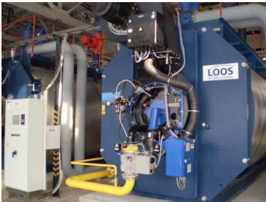
Fig.1. LOOS boilers, installed at the boiler-house Uvileyna str.,117 Artemivsk city (#152 in the project)
