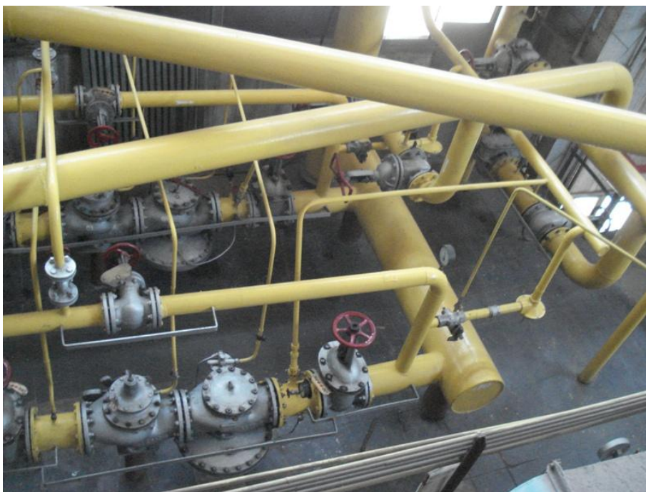
Fig. 2. Gas distribution unit
