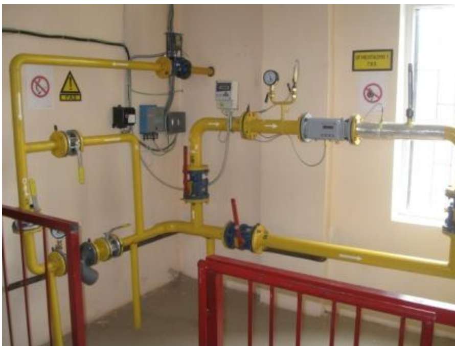
Fig. 3. Gas distribution unit
