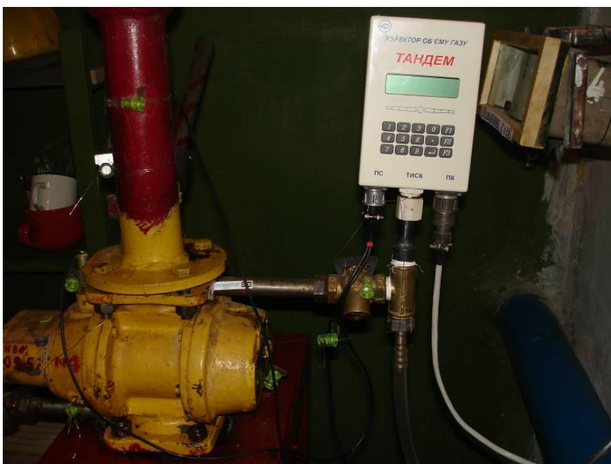
Fig. 4. Gas flow meter with corrector
