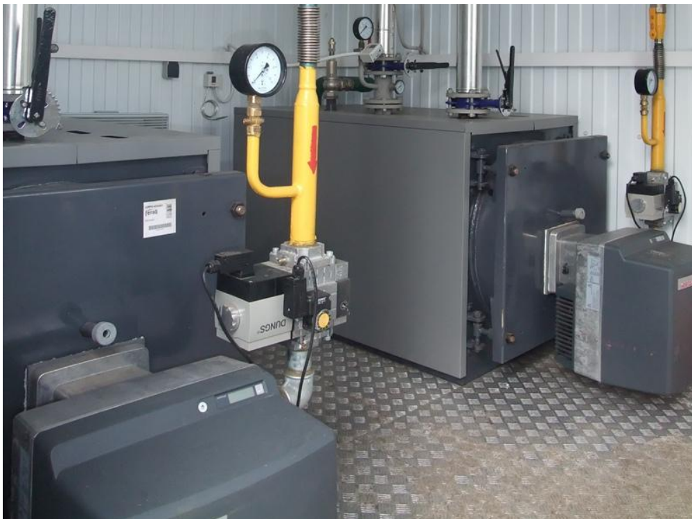
Fig.2. Modular boiler-house at Magistralnaya (#64 in the Project) with installed boilers KOLVI-550
