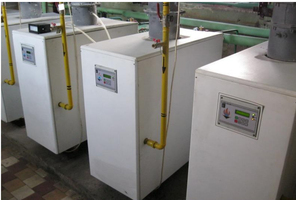
Fig. 1. New boilers OVK-100 LWE installed at boiler-house Pyatysotnitska, 19 (# 212)
