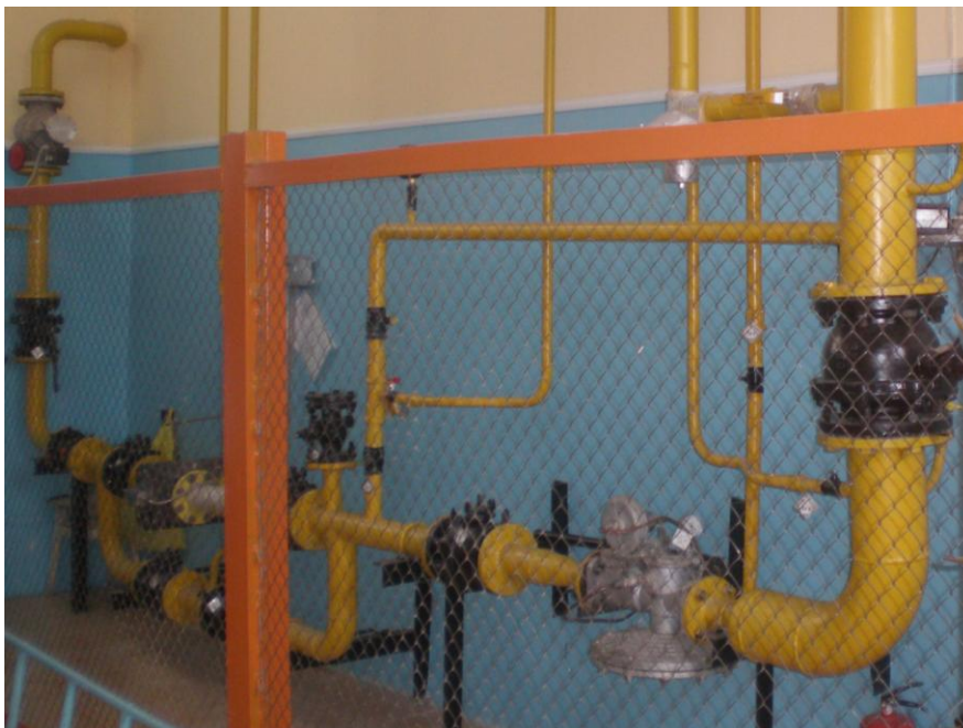
Fig. 2. Gas distribution unit
