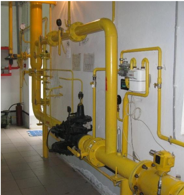
Fig. 3. Gas distribution unit
