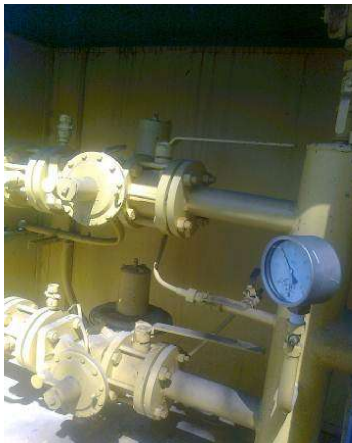
Figure 1. A repaired CGDP, Chernigiv
