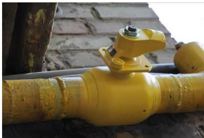
Pic.2 Ball valves DN80, register number 3944 (40-year of October avenue, 46-A)
