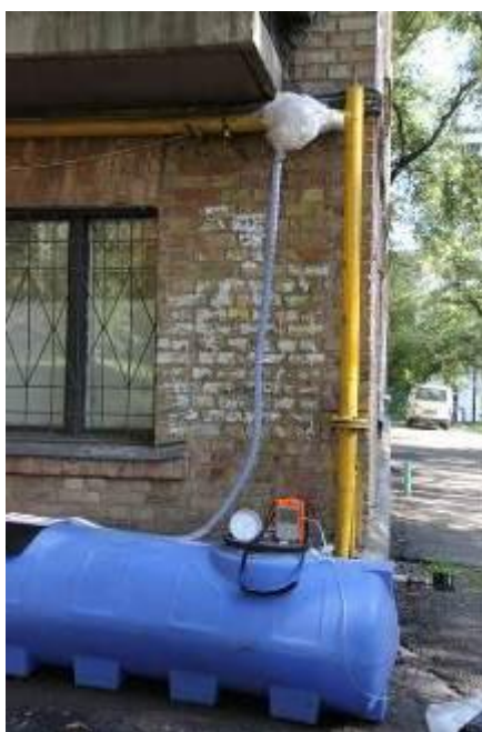
Pic. 4. Monitoring measurement of methane leaks on the ball valve, register number 3944 (40-year of October avenue, 46-A.
