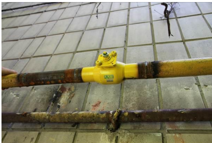
Pic.3 Ball valves DN50, register number 3927 (40-year of October avenue, 108/2)
