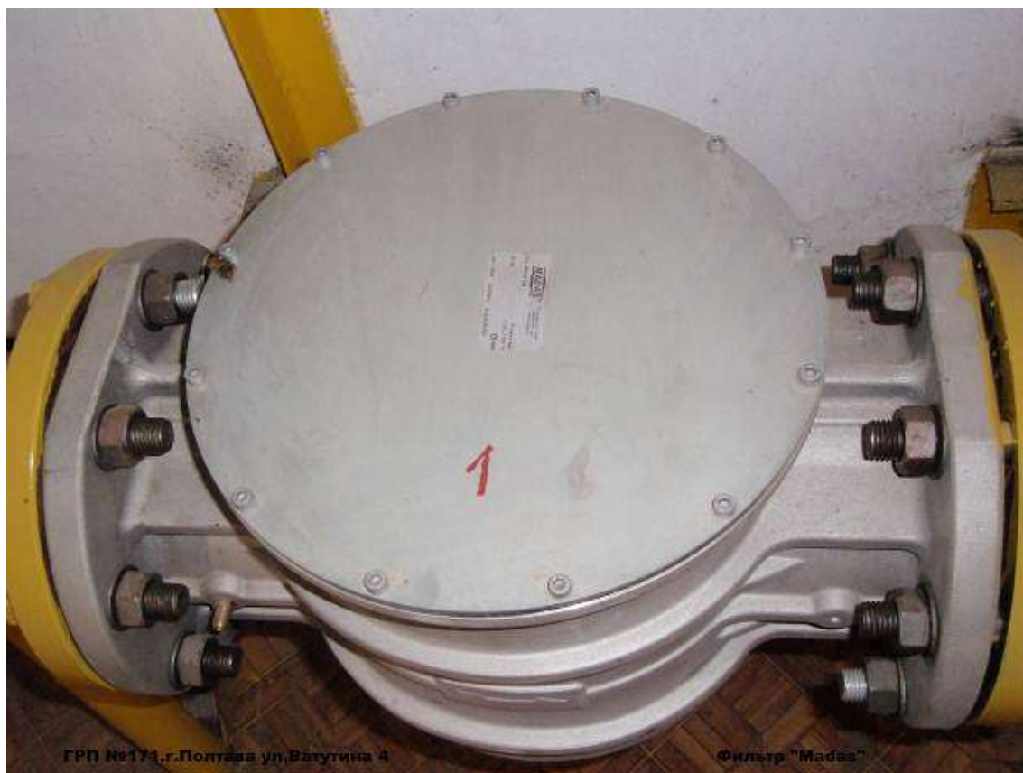
Figure 2. A replaced Madas filter at a GDP, registry No.434
