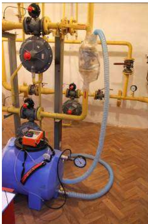
Figure 3. A device for quantitative measurement of methane leaks
