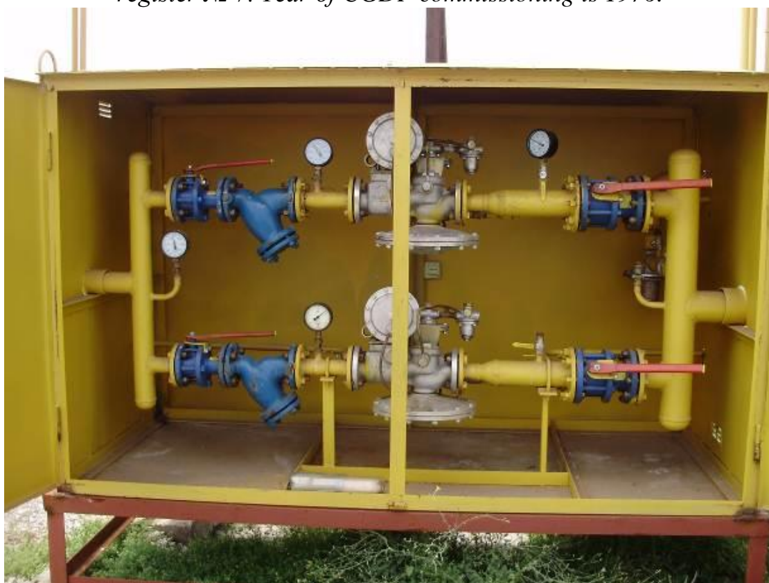
Pic. 2. Repaired CGDP in Kremenivka village, Chapaeva str., register № 80. Year of CGDP commissioning is 1982.
