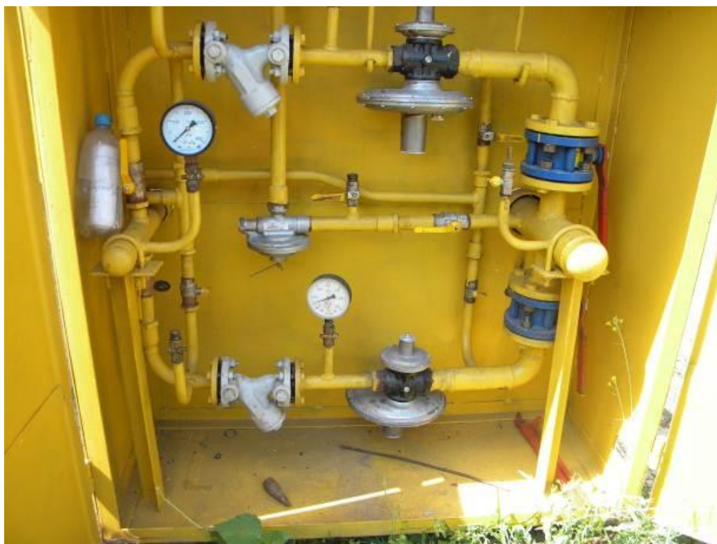
Pic. 1. Repaired CGDP in Mariupol city, Kulibina str., register № 7. Year of CGDP commissioning is 1976.
