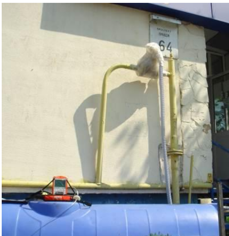
Pic.5. Monitoring measurement of methane leaks on wedge latch, registered number № 9945 (Avenue Pravda, 64)
