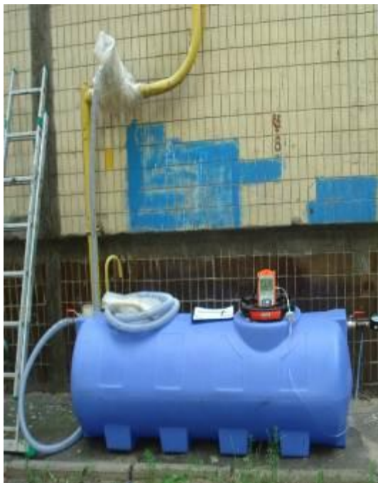
Pic. 3. Monitoring measurement of methane leaks on wedge latch, register number № 4020 (Marshall Jakubowsky str., 2A).
