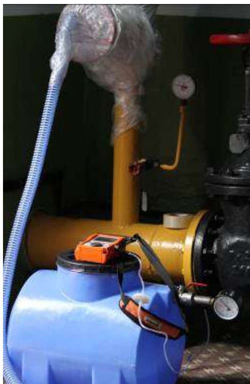
Pic. 1. Photo of quantitative measuring of methane emissions device.
