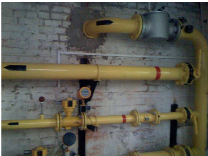
Fig. 2. Gas distribution unit
