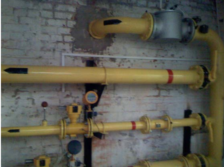
Fig. 2. Gas distribution unit
