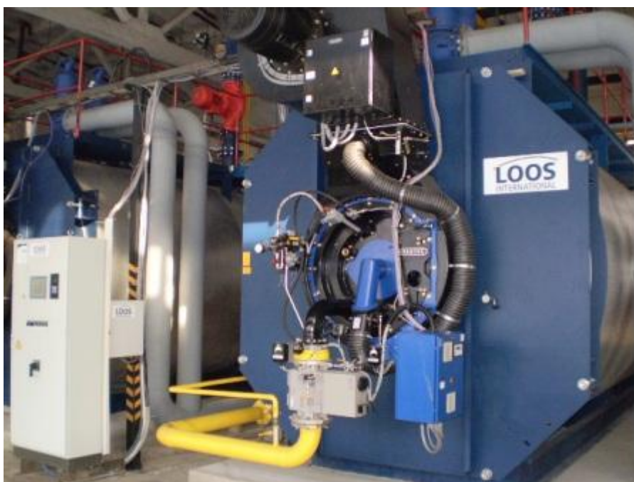
Fig.1 LOOS boilers, installed at the boiler-house Uvileyna str.,117 Artemivsk city (#152 in the project)
