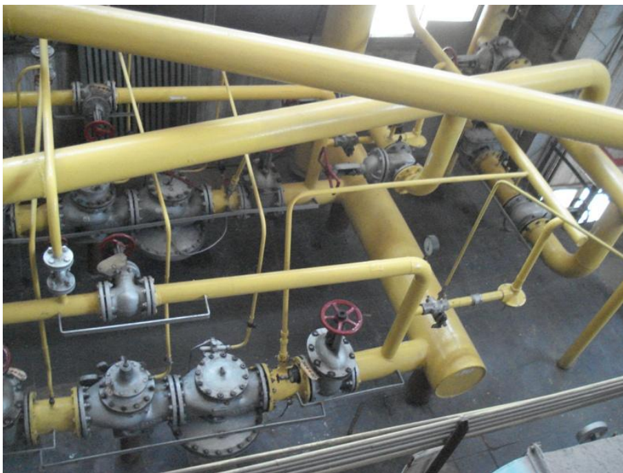
Fig. 2. Gas distribution unit
