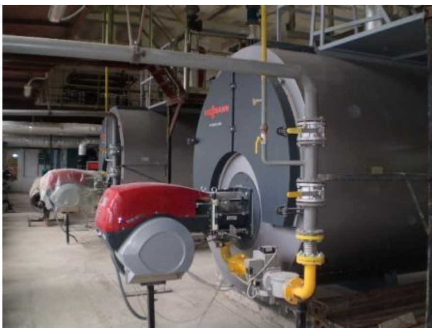
Fig.1 Viessmann boilers, installed at the boiler-house Karpinskogo str.,1-10a Artemivsk city (#155 in the project)
