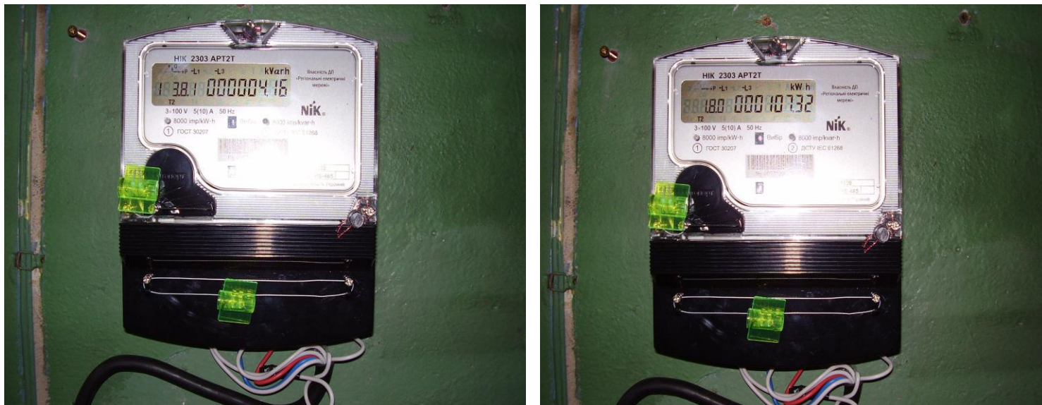
Figure 3 Electricity meter “NIK 2303ART2T”
