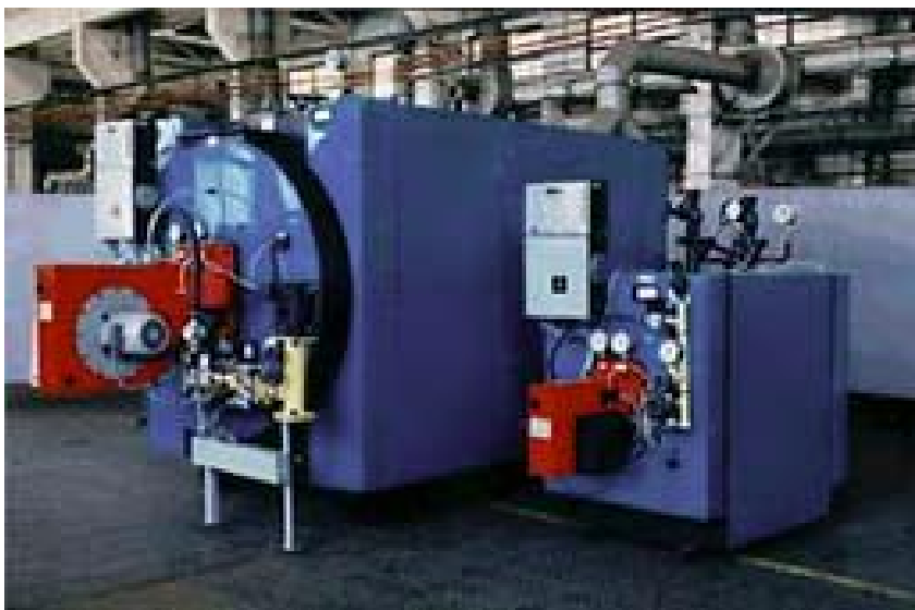
Fig. 3. The new boiler KSVa-1,25
