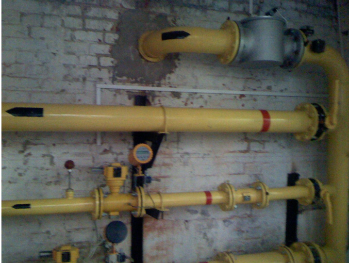
Fig. 2. Gas distribution unit
