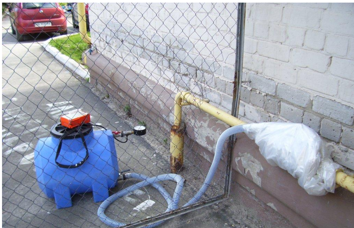
Picture. 1. Photo of a plant for quantitative measurement of methane leakage.
