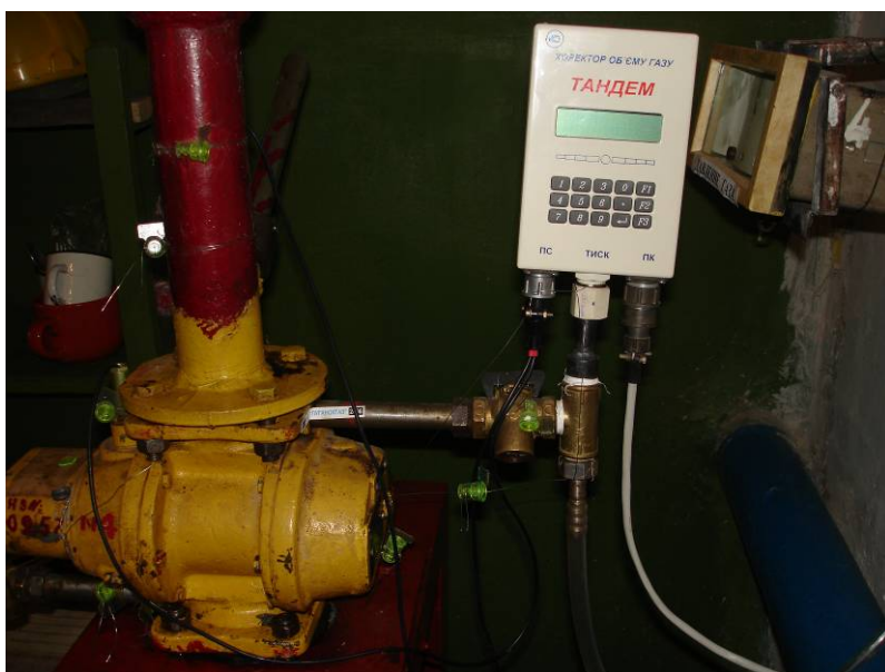
Fig. 2. Gas distribution unit
